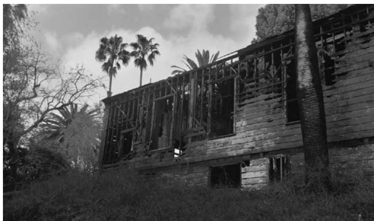
The results of the fire that destroyed the Little Country Church.
