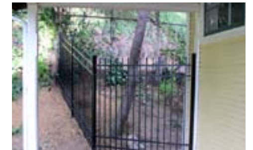
A new fence has been installed at the back end of the porch to protect the Lasky-DeMille Barn from transients who were using the area as a bathroom, causing a health problem. Funds for the fence were donated to the Hollywood Heritage Museum. Photo by Alan H. Simon
